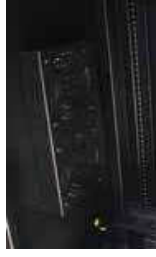
Fan units for dissipate heat
